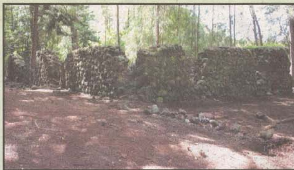
After the clean-up, all of the debris was hauled away, leaving everything neat and tidy.
